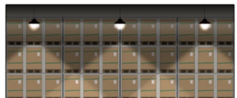
Many LED high bay present light with significant drop off between fixtures and a dark background.
